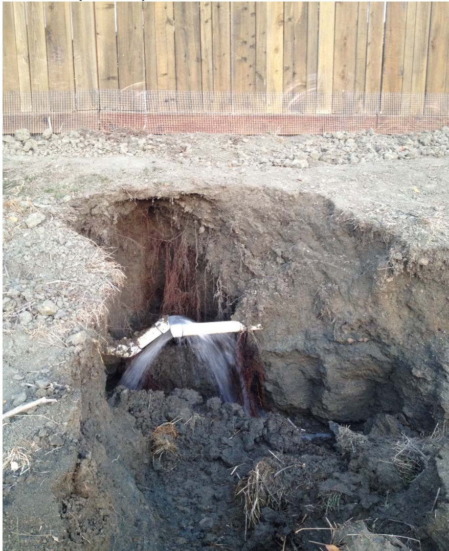
FIGURE 1: Permanently pressurized irrigation line break on slope immediately downslope of residence
