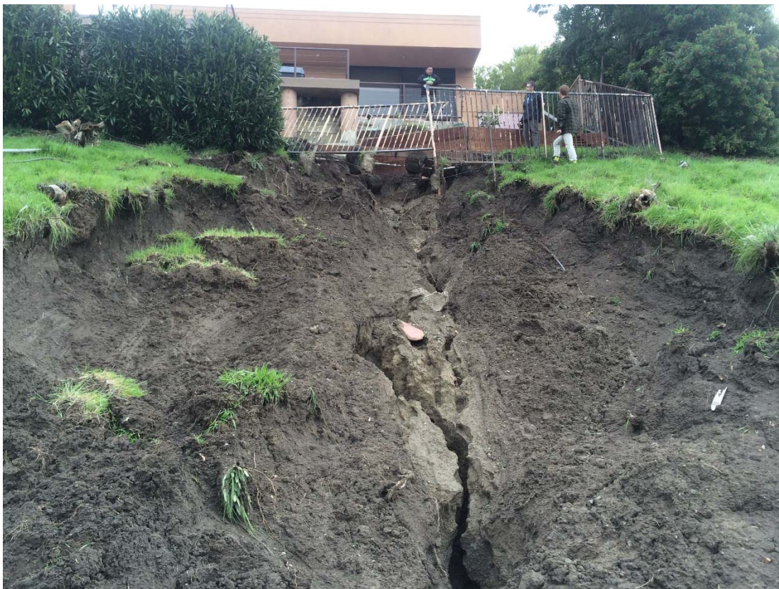
FIGURE 2: Landslide below residence located at the top of slope. Note broken white irrigation pipe at top of landslide downslope of wood retaining wall.
